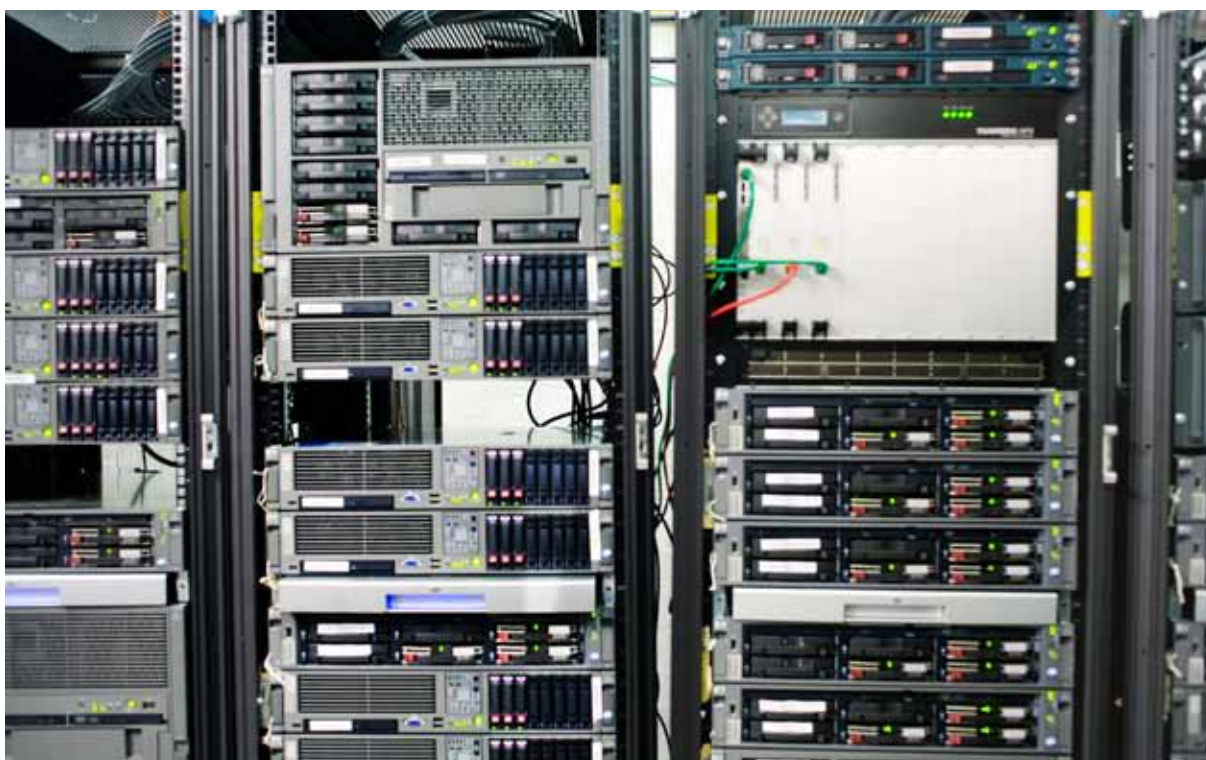
Server stack at ECDC
